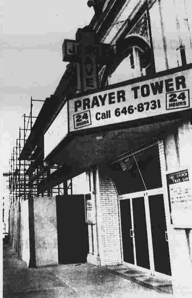
The familiar yellow marquis will remain the same, but the rest of the Full Gospel Interdenominational Church on Main Street is getting a facelift. Workers are currently scrubbing the brick front of the building and replacing mortar. On the inside, space which the church used to rent to shops and a law firm is being converted to classrooms and a "children's church."
